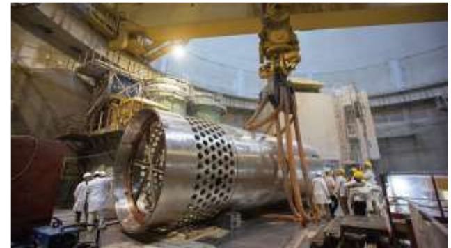
Work to install Rooppur 1's core barrel was completed in May 2023 (Image: Rosatom)
