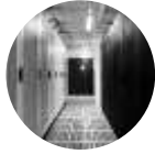
Power Storage Units
