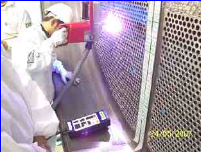
Tube to tubesheet welds
